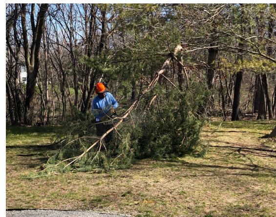
(Top to Bottom) Volunteers work on the biocell on the UUS campus, Gary Lawrenson and Pete Brokaw worked on the flat roof, Pine tree limbs are trimmed and removed.
